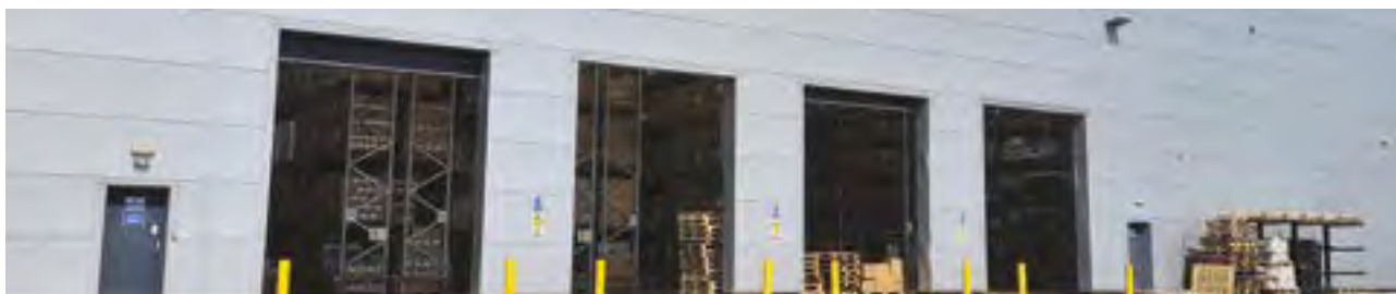
Uncontrolled ventilation can result in higher energy demands
